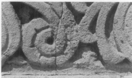
Cracking of limestone. Photograph: John H. Myers.
